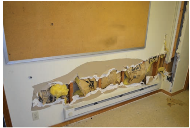
FIGURE 65. DETERIORATING PARKS M&O FACILITY
