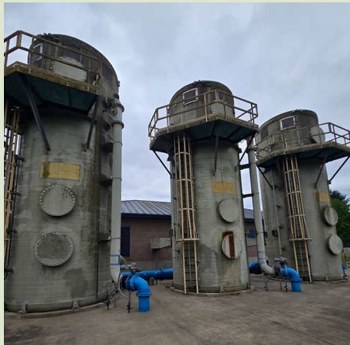
Fulmer Treatment Facility
