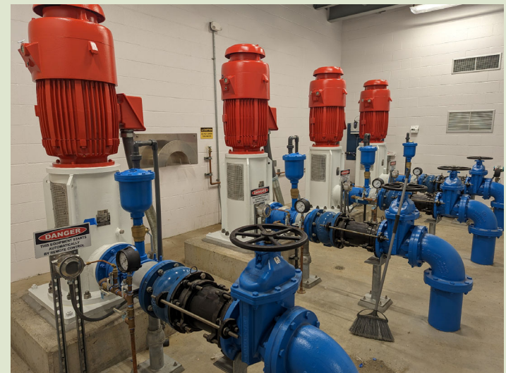
Academy Pump Station
